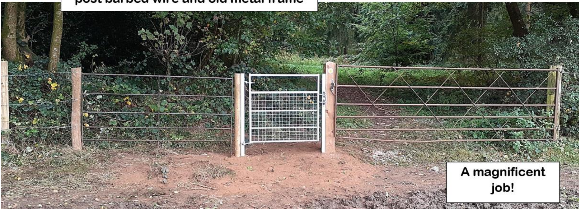
Final tamping down; replacing the soil, post barbed wire and old metal frame
